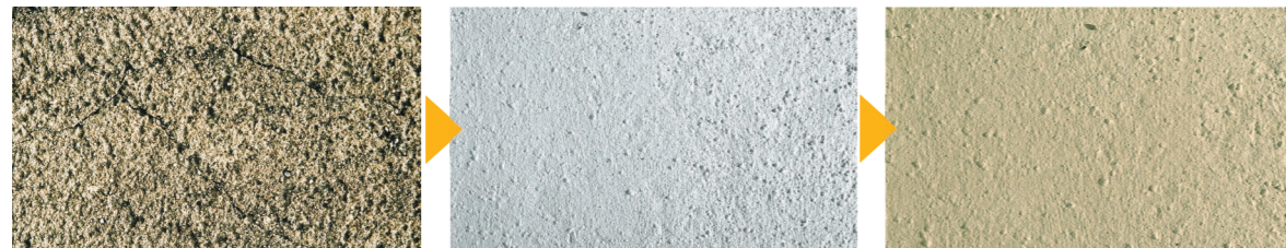
Existing render with cracks
