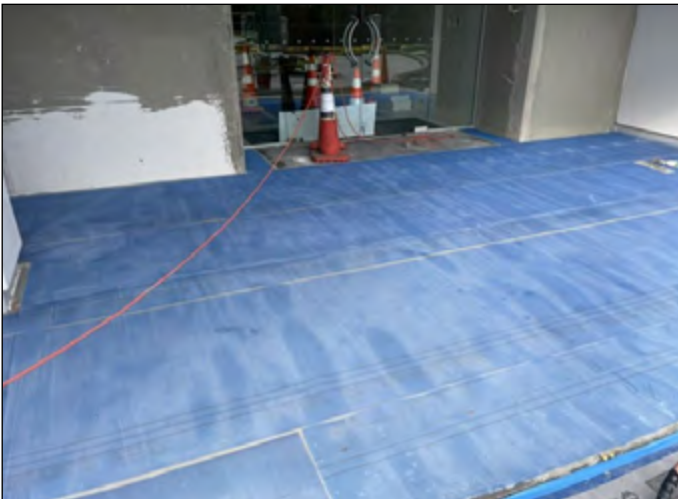
Textile antifracture mat installed as a decoupling layer over the Matacryn membrane
