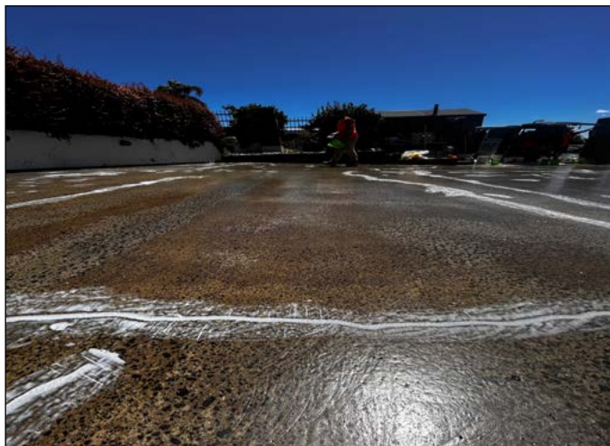
The prepared concrete is primed with Matacryl 108 H primer and then the cracks are repaired using Matacryl LM
