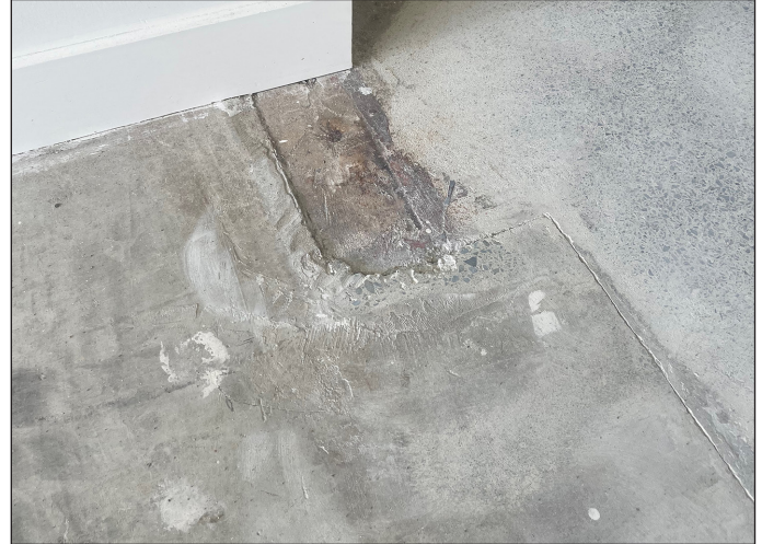
Existing garage floor, with a mix of old and new bare concrete
