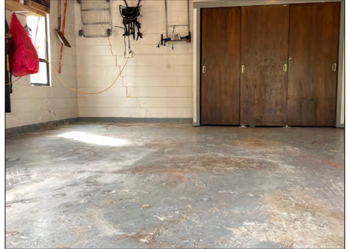
Existing coating lifting due to wear from car tyres
