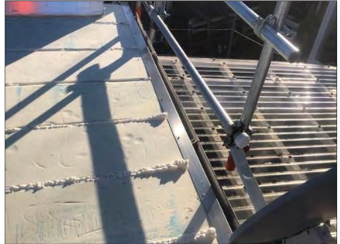
Installation of XPS infills glued between the metal ribs to provide a base for the PIR to be installed
