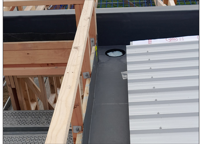
The FLAGON TPO 90 degrees external corners are in place for extra reinforcing and stability
