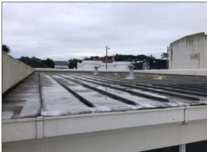
Original iron roof
