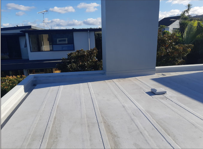
Original roof with old membrane
