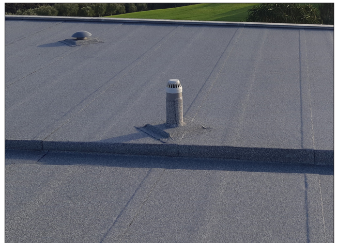
Pipe penetrations and short roof vent on plinths
