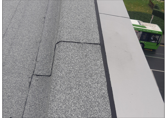
Alsan Mastic 2200 sealant to seal DUO cap sheet against aluminium parapet capping
