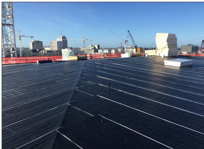
Steel roof with vapour barrier applied ready for PIR thermal insulation board installation
