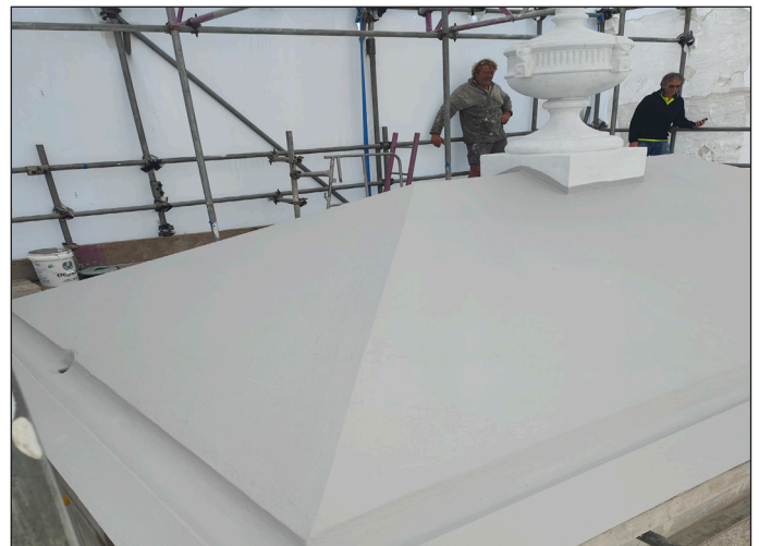
Chevaline Dexx system was used on all flat/low pitched surfaces including roof, internal roof and parapets
