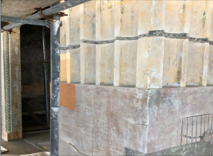
Earthquake damaged concrete
