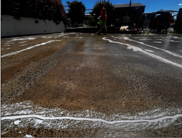
The prepared concrete is primed with Matacril 108 H primer and then the cracks are repaired using Matacril LM
