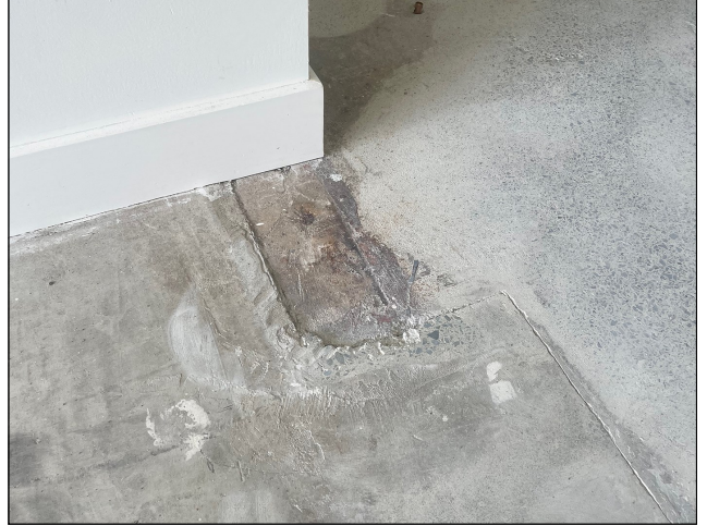
Existing garage floor, with a mix of old and new bare concrete
