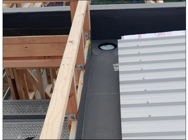
The FLAGON TPO 90 degrees external corners are in place for extra reinforcing and stability
