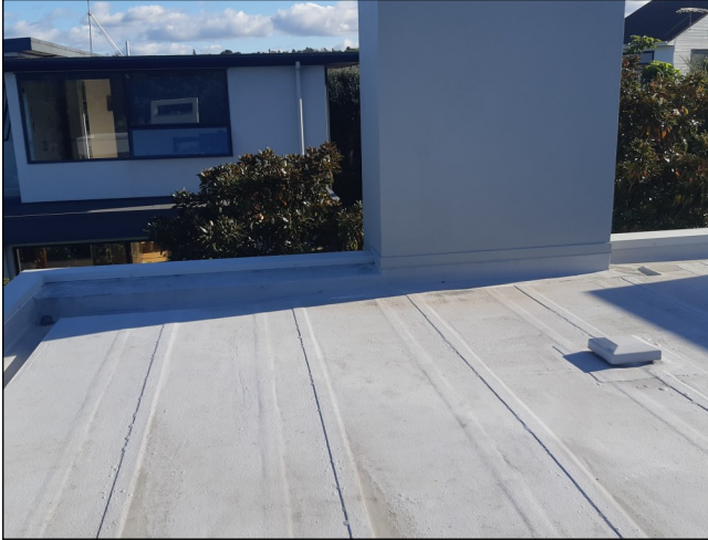
Original roof with old membrane
