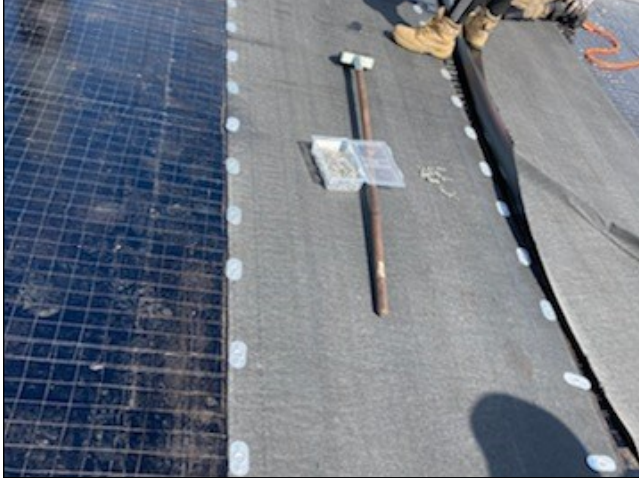
Mecano fixing plates with screws at 150mm spacings to mechanically fasten the Deboplast basesheet
