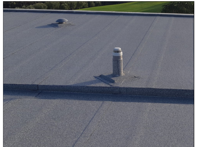
Pipe penetrations and short roof vent on plinths
