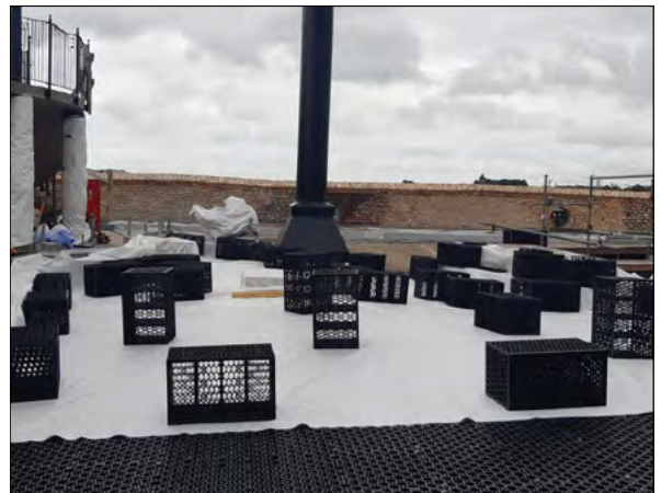
Drainage cell installation over Duo Landscape membrane before the green roof installation
