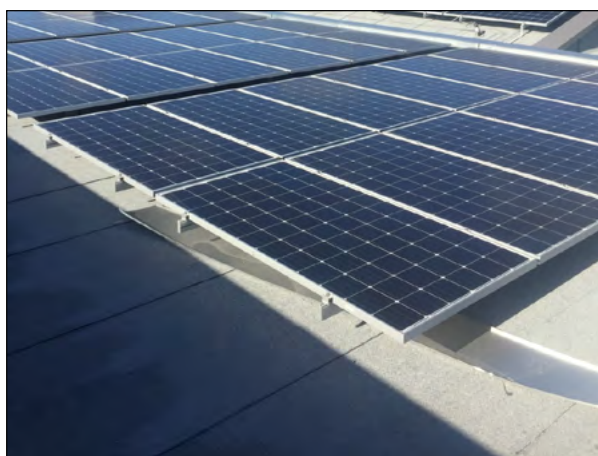
Finished project with PV Panels installed
